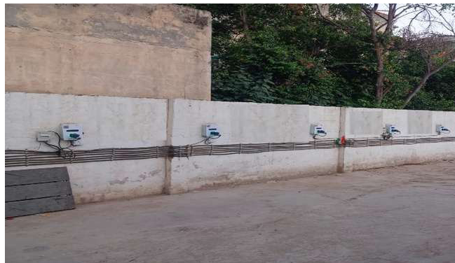
Fig 6: Deployment of LEVAC Charger at E-Rickshaw Hubs
