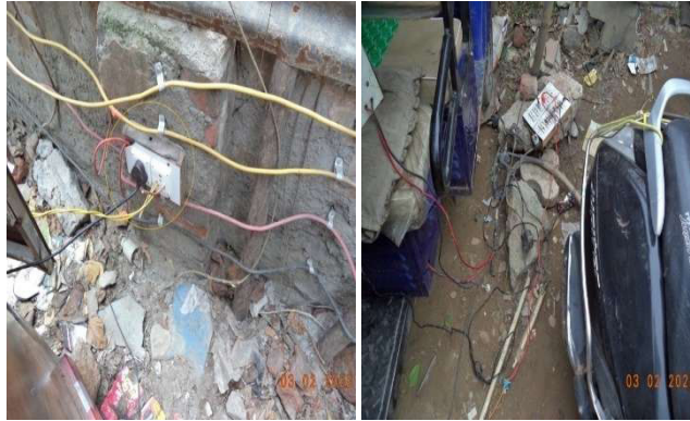
Fig 4: Unsafe output Plug Points at ERCH
