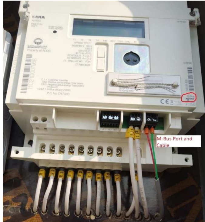
Fig. 4 M-Bus cable connected using M-Bus port of electricity water on the field
