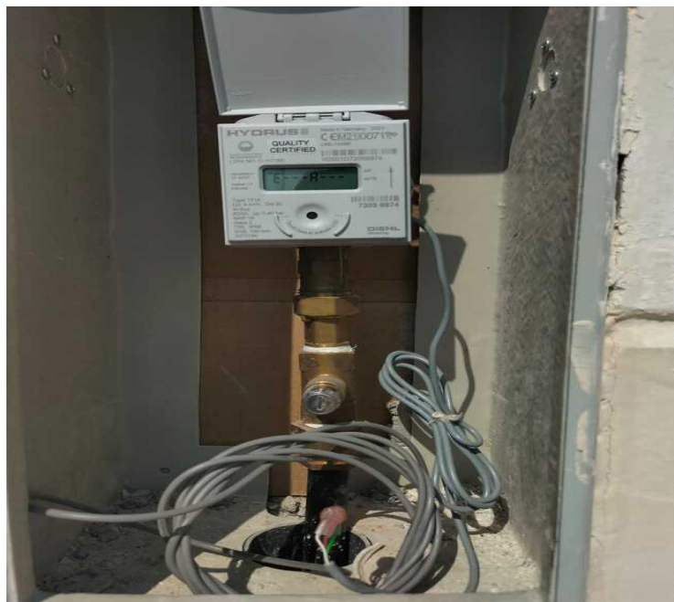
Fig. 5 M-Bus cable connected to water water on the field
