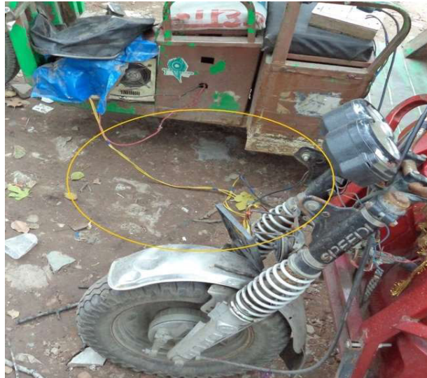
Fig 5: Unsafe Wiring at ERCH
