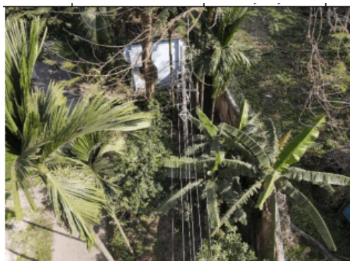
Fig. 4: Plot of overhead conductors with significant amount of Sag
