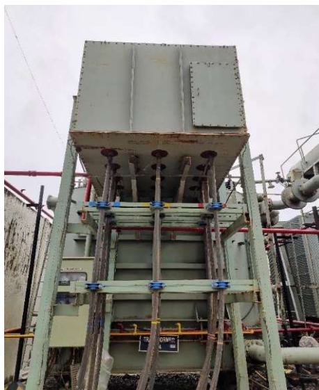
Fig.1: Transformer LT Cable Box
