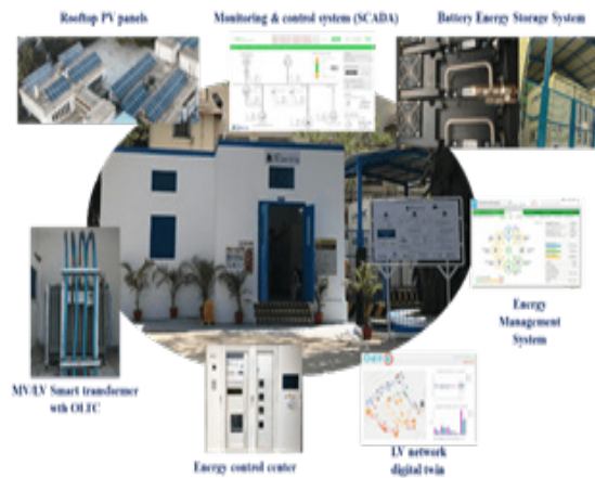
Fig.1 Shakti on site final set-up
